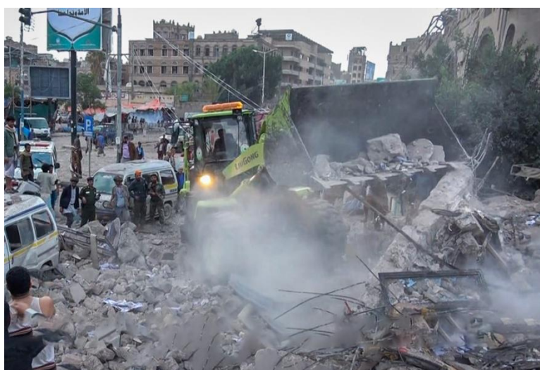
Some of the destruction caused by the Israeli airstrikes on Al-Tahrir neighborhood, Sana'a, 10 September 2025
